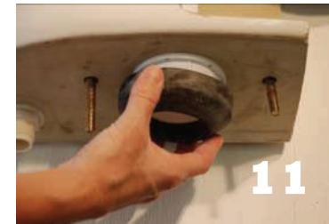
11 Replace tank seal.
